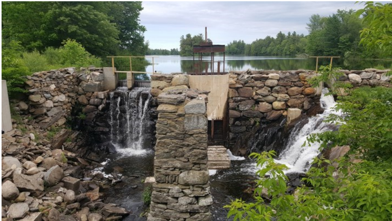
Dam at Branch Pond that is slated for removal to return fish passage routes
